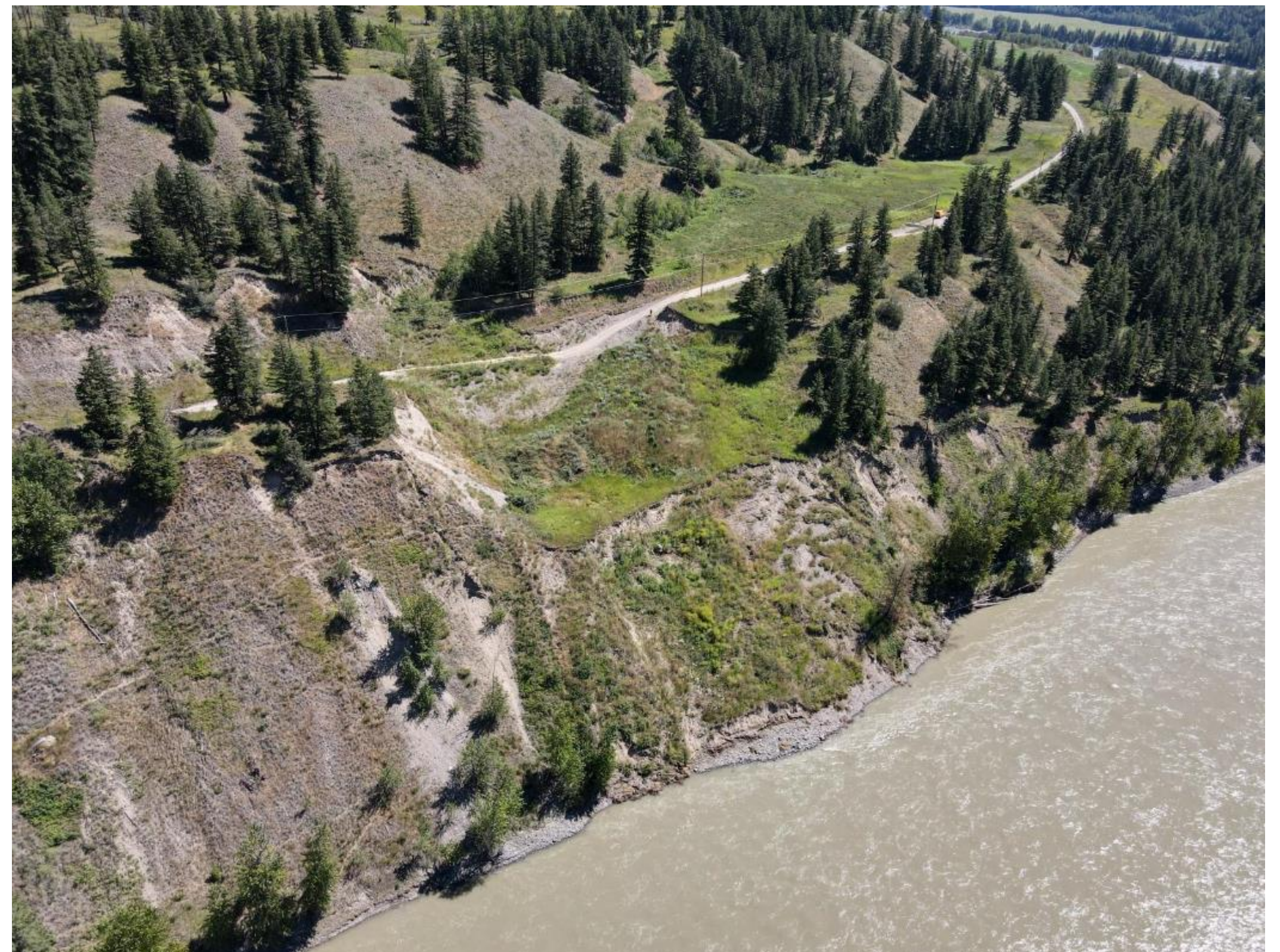
Aerial photo of the slide site, with the Fraser River in the foreground. Photo from summer 2022.
